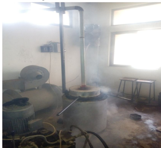
Fig. II furnace being heated
