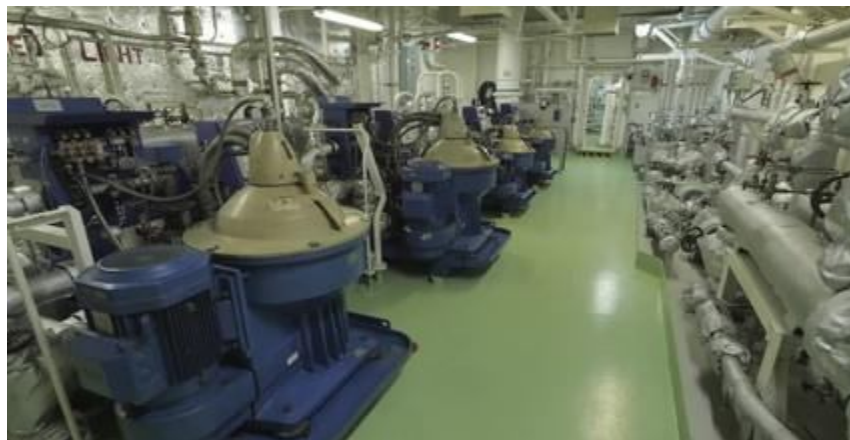
Fig 1: Centrifugal fuel oil separators[1]
