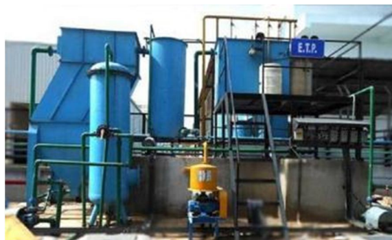
Fig.2. An Effluent Treatment Plant
