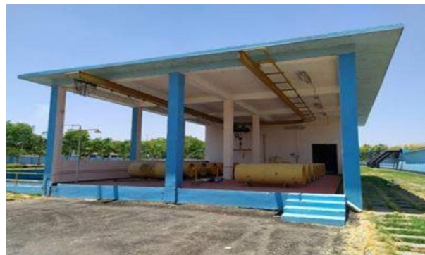
Fig.12. View of Chlorination unit
