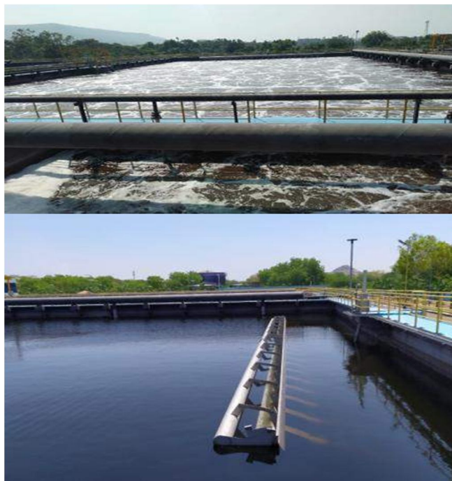
Fig.8. View of Aeration and Decanting
