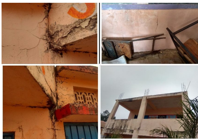
Fig.1 Defects in Jivan Salashi
