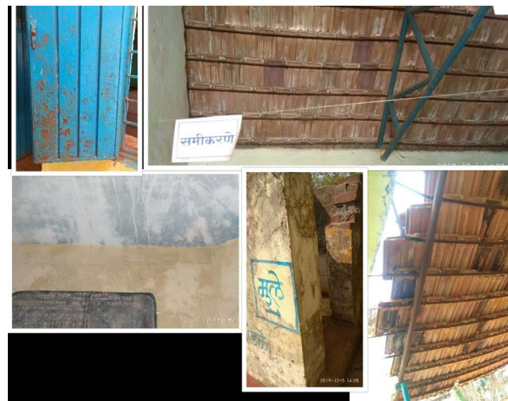
Fig.3 Defects in Bhadale
