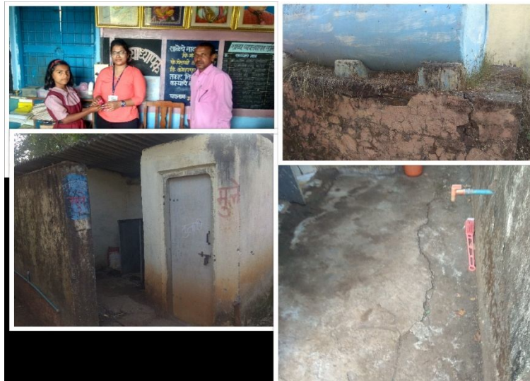
Fig.4 Defects in Vhanagdewadi
