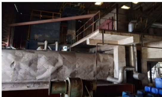
Fig 2: Briquette Boiler in Plant
