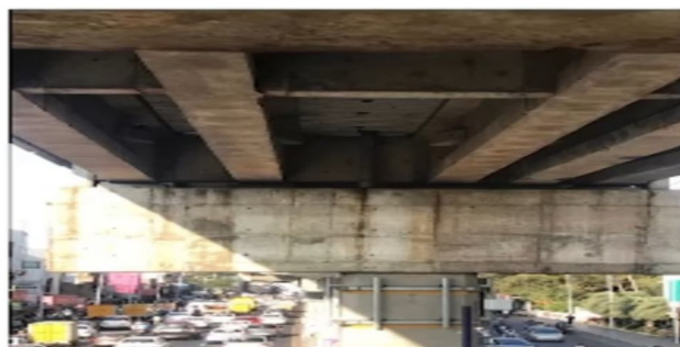
Fig 2: shows the a real bridge structure which is prone to carbonation attack.
