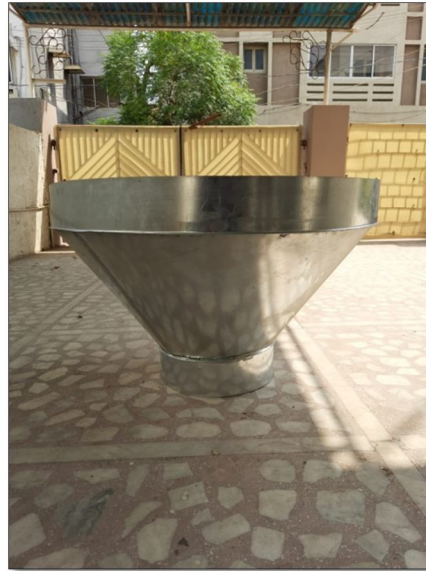
Fig 19: Divergent duct fabrication
