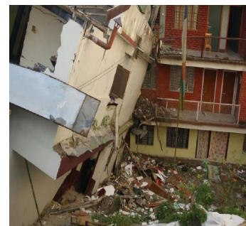
Fig 3 Sikkim Earthquake Caused Collapse of Government Building
