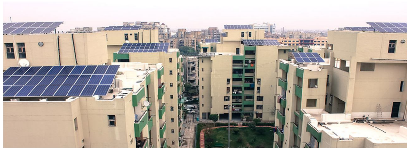
Fig 2 roof top solar system
