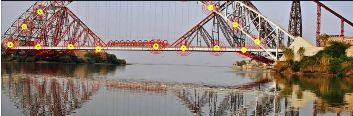
Fig. 1 Structural Health Monitoring with sensors on a Bridge
