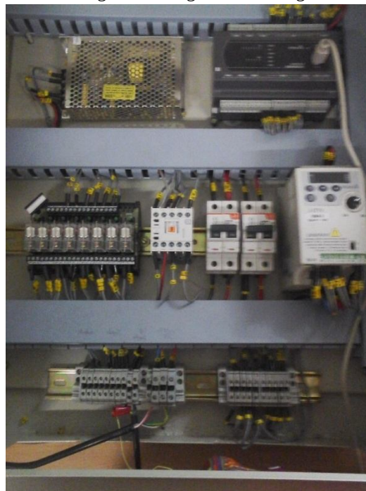
Fig 3.: PLC Panel Board
