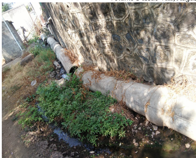
Fig.2 Poor Sewage Disposal System in kondave village
