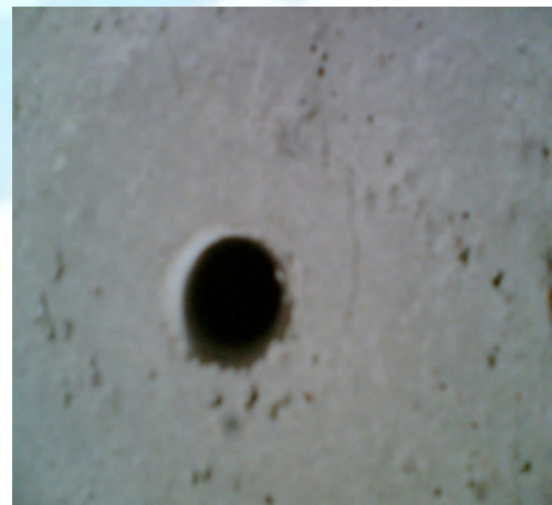
Fig. Hole in the brick
